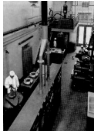
Figure 48.4. Plant for the fabrication of uranium dioxide ( UO_2 ) pellets. Picture shows equipment for powder preparation, a hydraulic press, a sintering furnace (lower left), and pellet grinding machines (right).
